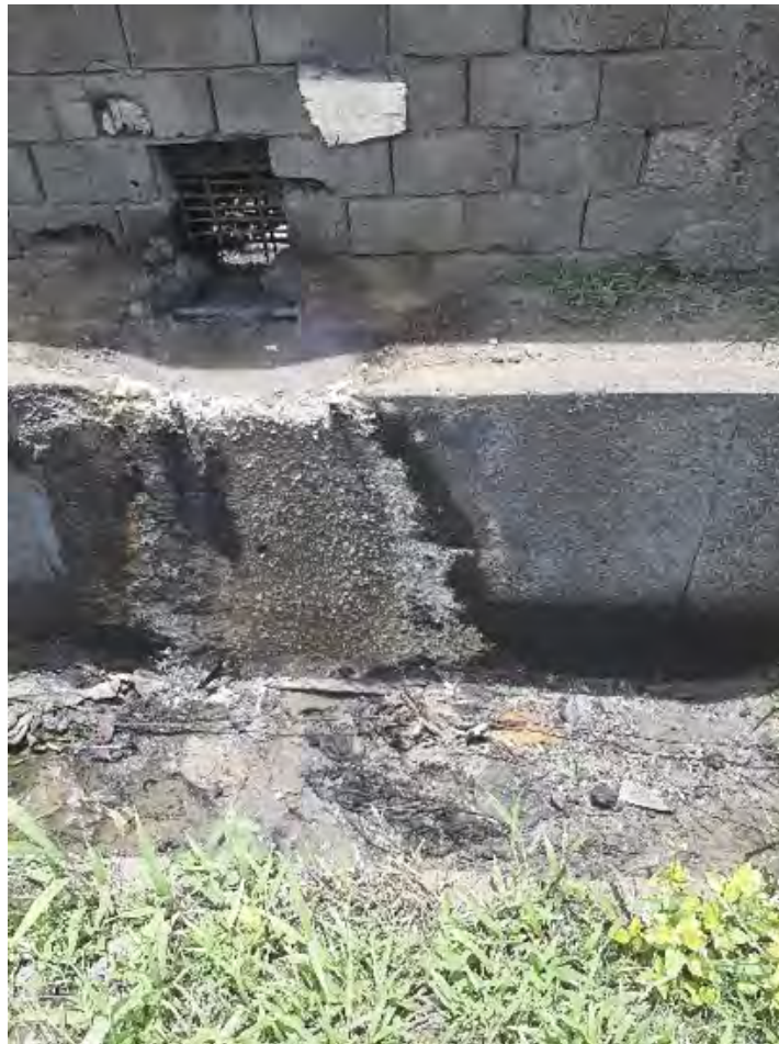
Figure 4. Untreated effluent discharged into an adjacent residential area outside of METAFRIQUE Cameroon SA. Note the corrosive effect of the acidic effluent on the concrete.
